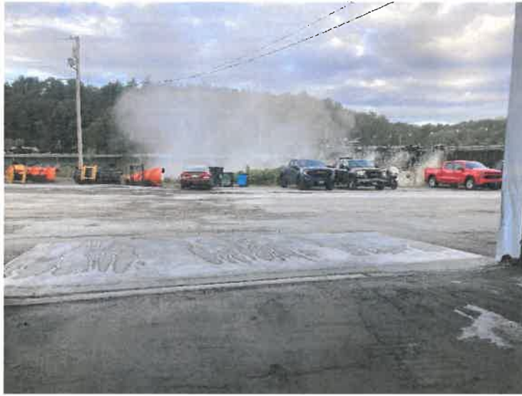
Photo 9. Looking west out of salt shed. Mist/vapor is coming off the Lamoille River, immediately below the outfall from the Arrowhead Lake dam. The dam is on the right. The grade off the parking lot is toward the river.
