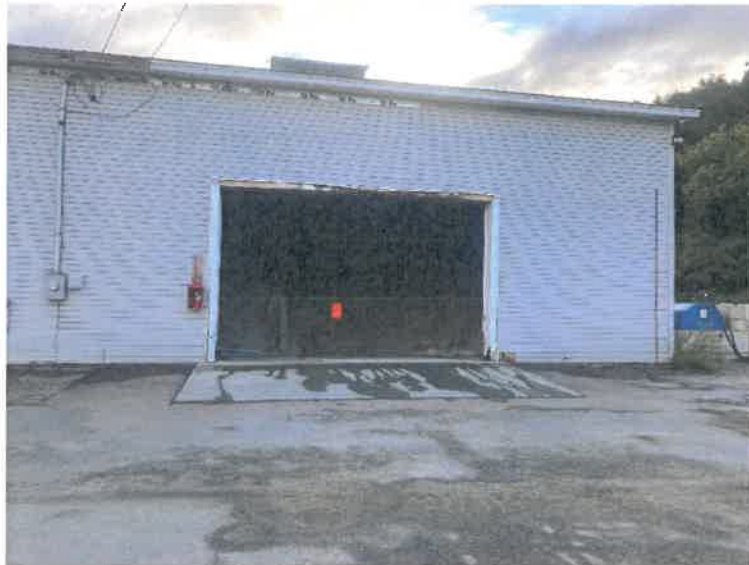
Photos 2. Salt shed bay. Door is too small, resulting in the frame commonly getting hit. Delivery trucks can't get completely inside the shed. Fuel tank on the right, outside the building. This bay has a 400 ton capacity.
